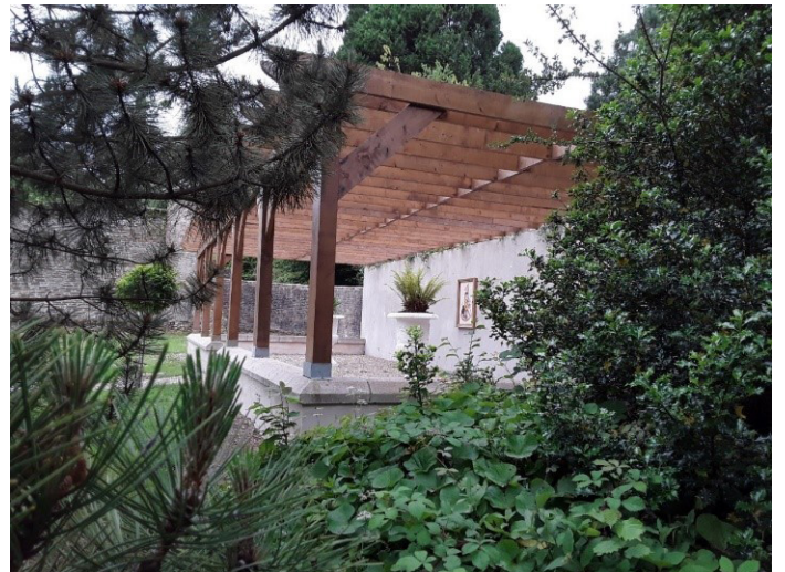
Newly completed pergola with plaque acknowledging the Tighe Estate the original owners of the Woodstock Estate
