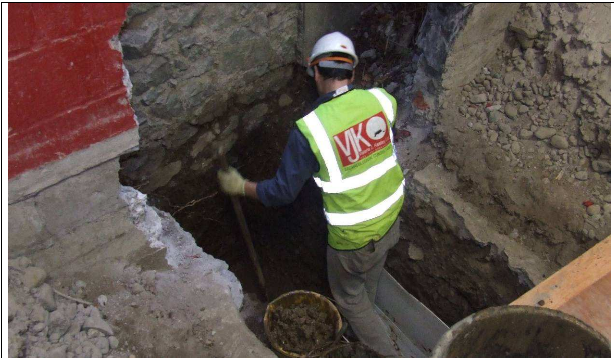
Plate 7: Trench VII following removal of 2 nd floor and concrete ring-beam under block wall C60. Looking south.
