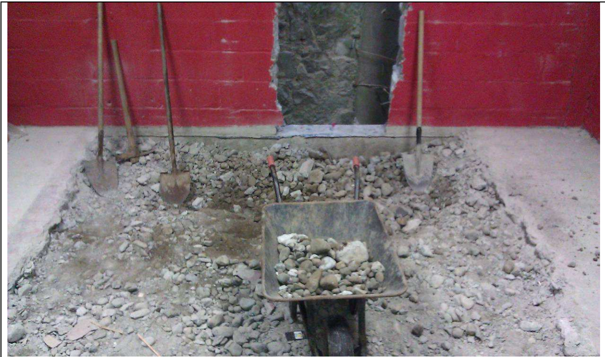
Plate 5: Trench VII showing initial removal of concrete floor and new opening in block wall. Looking southeast.
