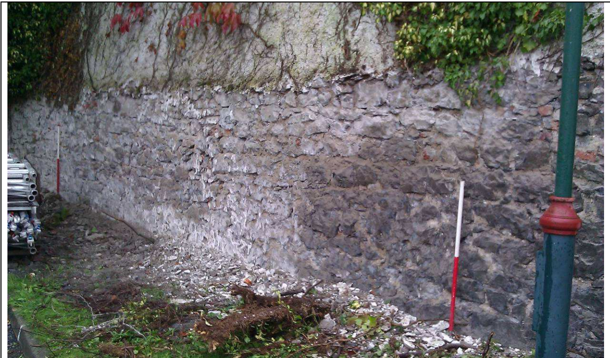
Plate 1: View of masonry wall C01 with pebble-dash removed, from Collegetown looking southwest.
