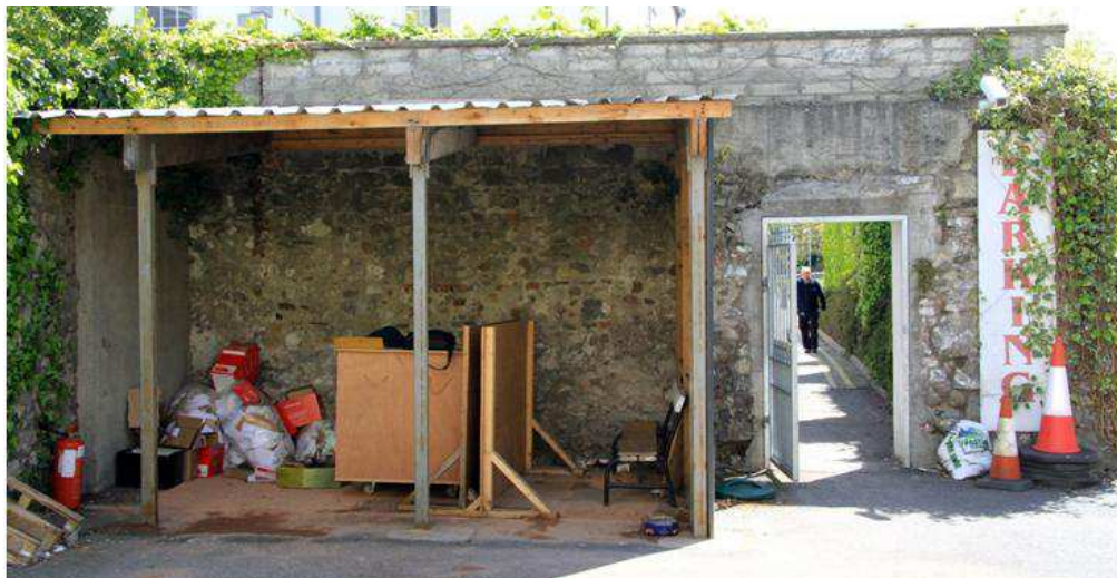
Plate 8: Rear boundary wall of number 75 John Street Lower
