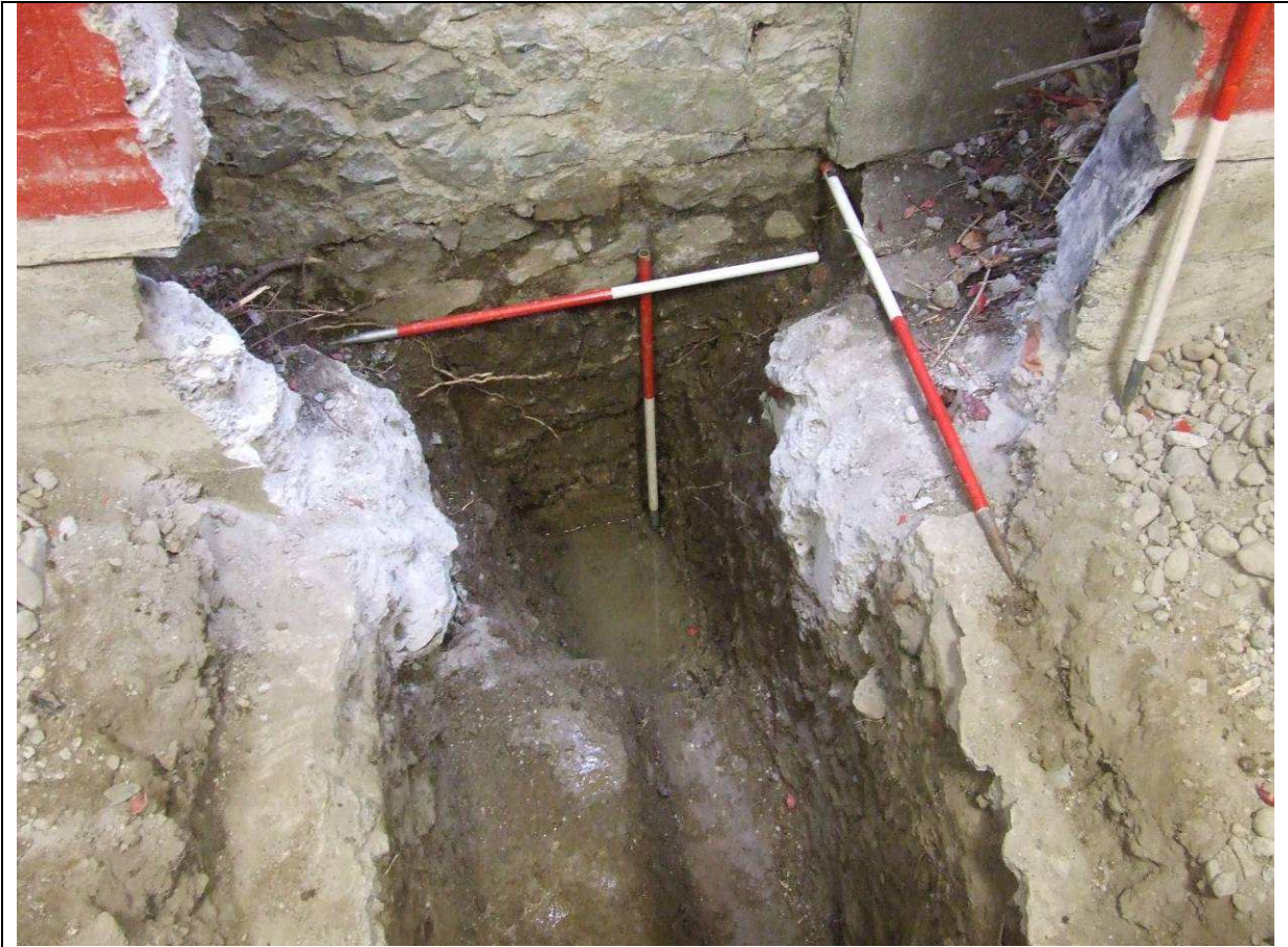
Plate 9: Trench VII, showing water-table, lower masonry wall C01, and archaeological deposits C65 (mortar) C66 (sticky clay) and C67 (fluvial clay), looking south.
