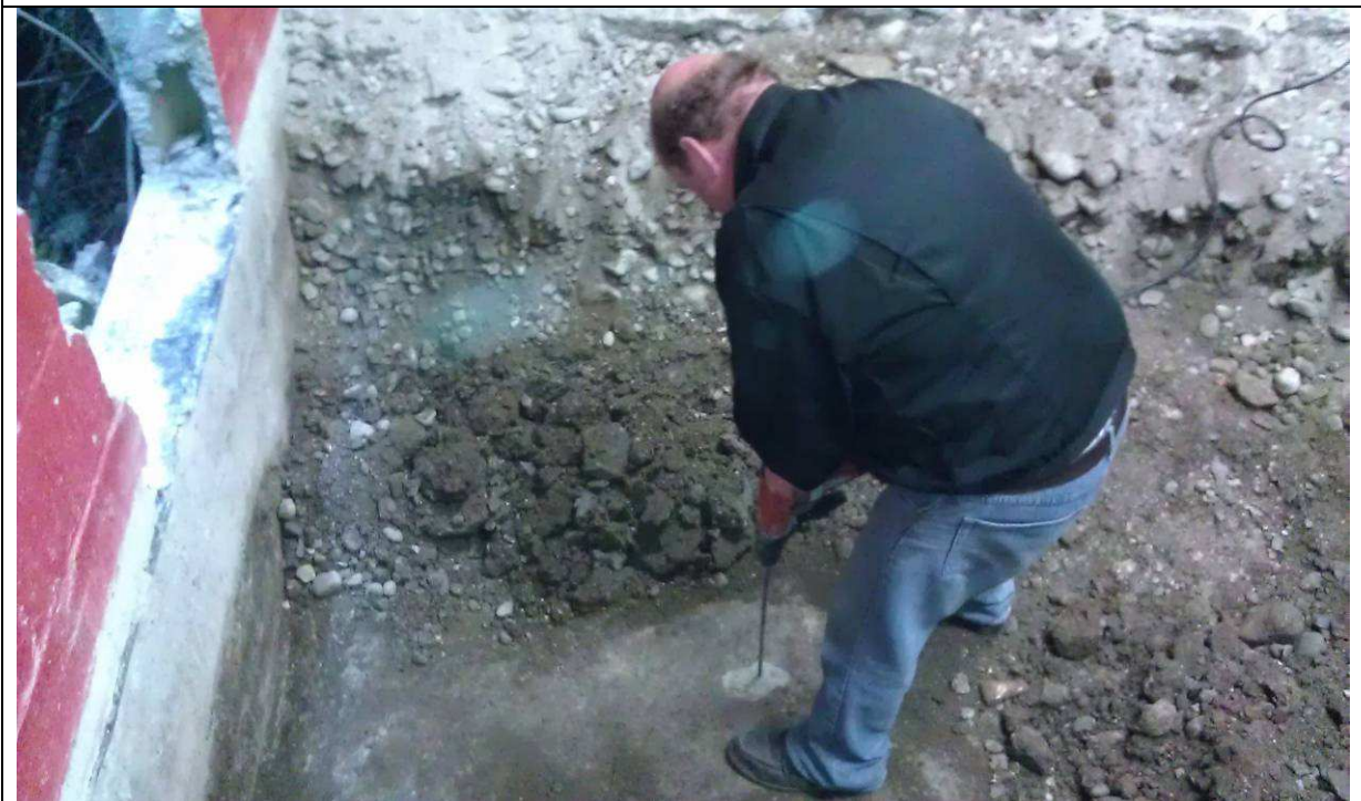
Plate 6: Trench VII in progress showing 1m of modern overburden over 2 nd concrete floor. Looking south.
