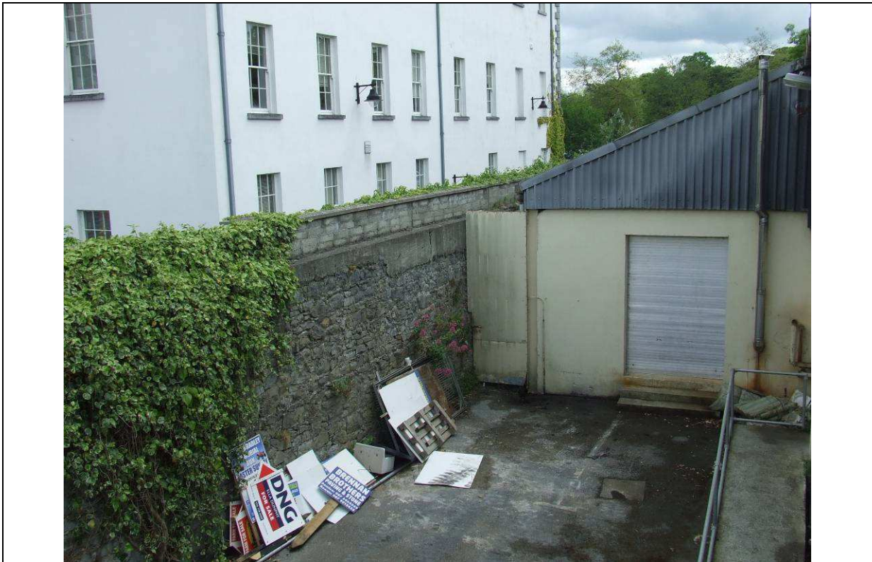
Plate 10: Boundary wall C20, view from rear no. 76 John Street Lower (Gardens townland), looking east.
