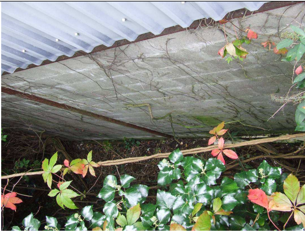
Plate 4: View of external southeast wall of Arts Building adjacent to heavily overgrown masonry wall from above.
