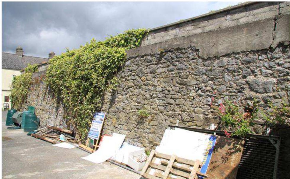
Plate 9: North-eastern side boundary wall of number 76
